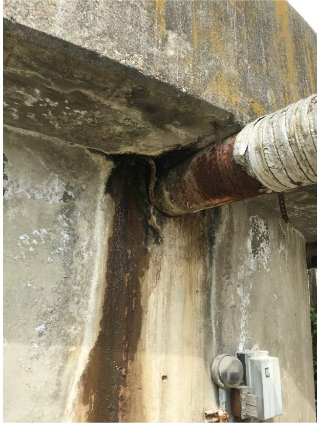
Figure 29. Leaking pipe at north-most sludge thickener.
