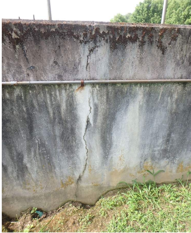
Figure 23. Typical crack at secondary clarifier.
