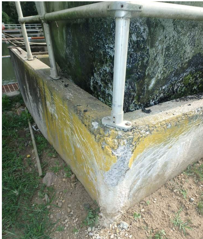
Figure 24. Spalling concrete at guardrail anchorage at secondary clarifier.
