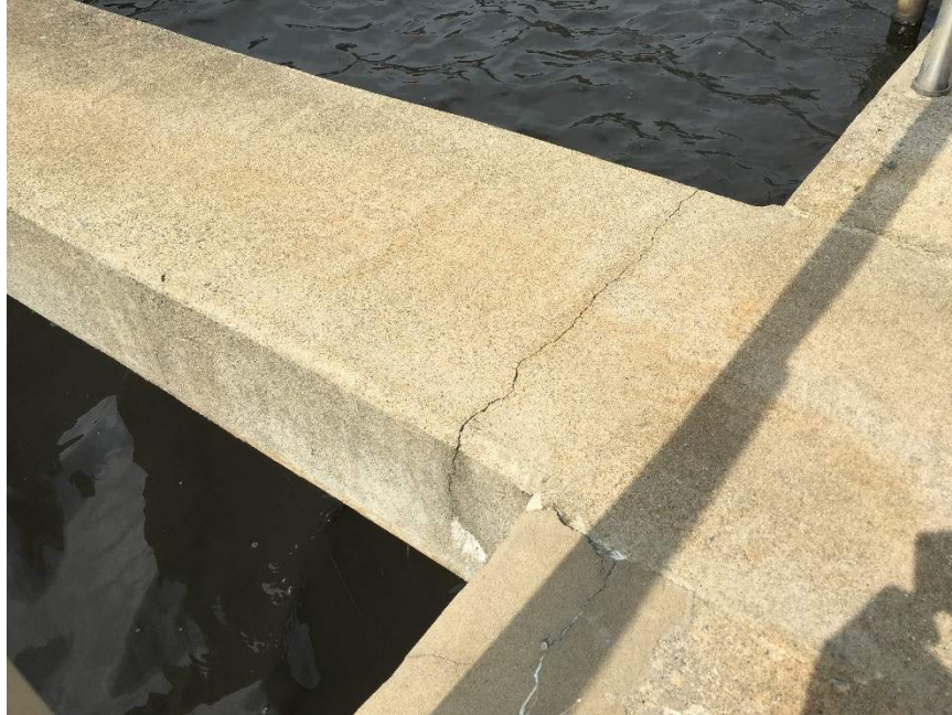
Figure 15. Minor flexural crack and delaminating concrete at horizontal brace.
