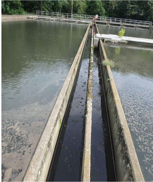
Figure 21. Central rough at secondary clarifier.
