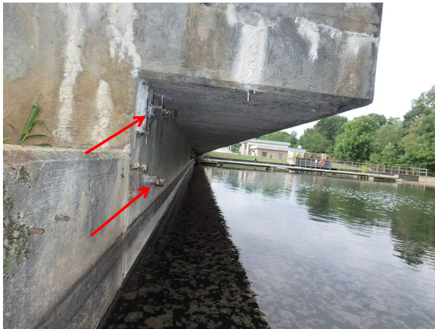
Figure 10. Anchor rods (red arrows) installed as retrofit presumably intended to arrest excessive lateral movement of west perimeter wall of aeration basin.
