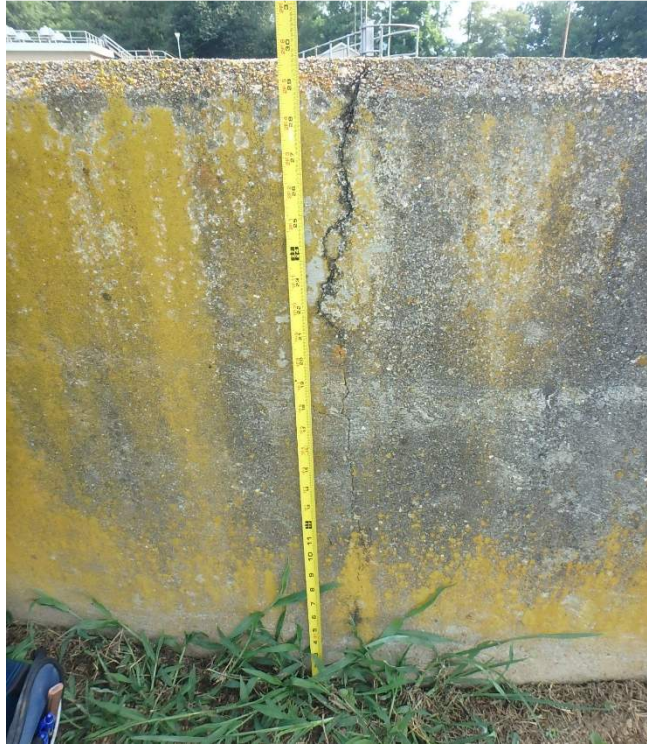
Figure 5. Crack at primary clarifier with minor leakage.
