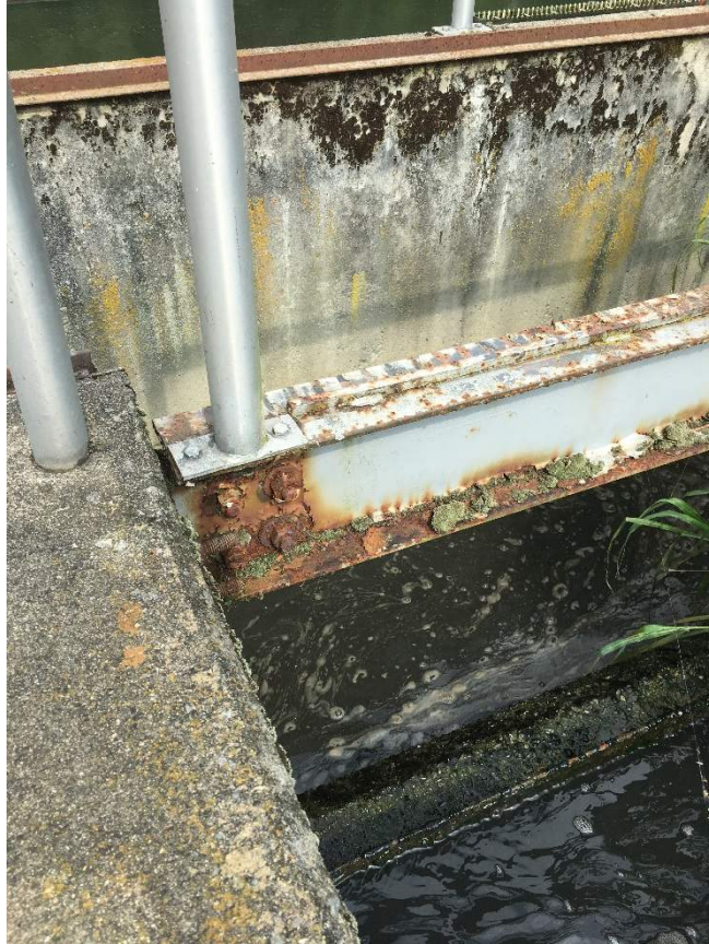
Figure 19. Corrosion at steel beam at embedded plate connection.
