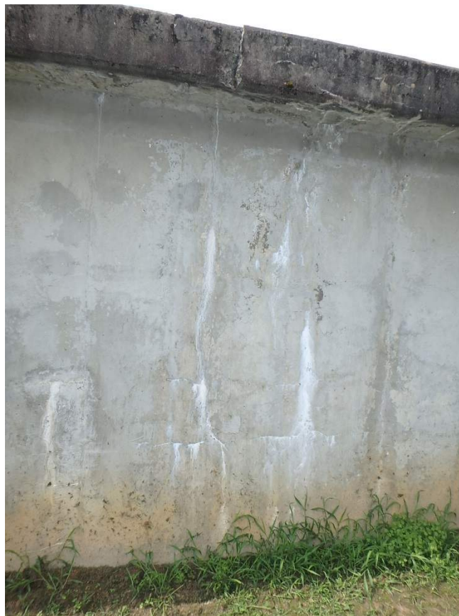
Figure 12. Typical cracks with efflorescence at north perimeter wall of aeration basin
