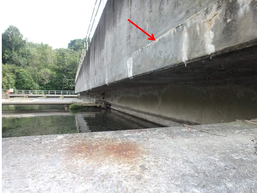
Figure 13. Continuous horizontal crack and efflorescence (red arrow) indicate seepage through cold joist at drainage trough wall.
