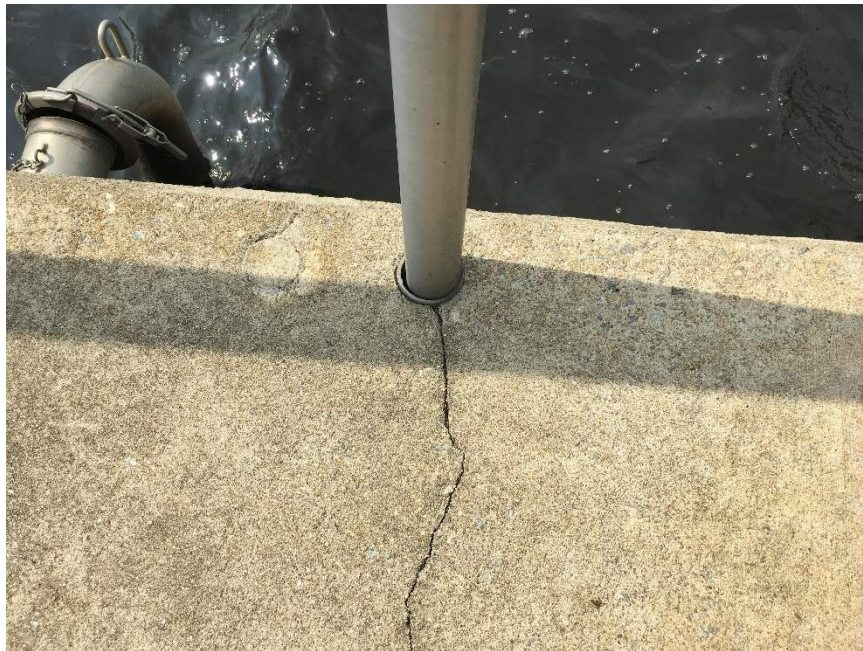
Figure 16. Freeze-thaw cracking at guardrail post penetration.
