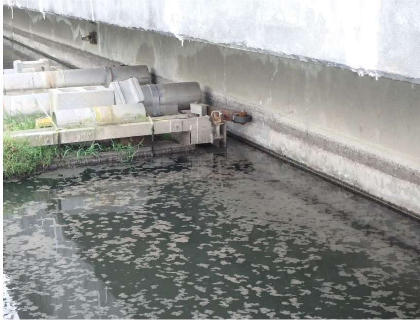
Figure 25. Abraded concrete along path of skimmer arm guide wheel.
