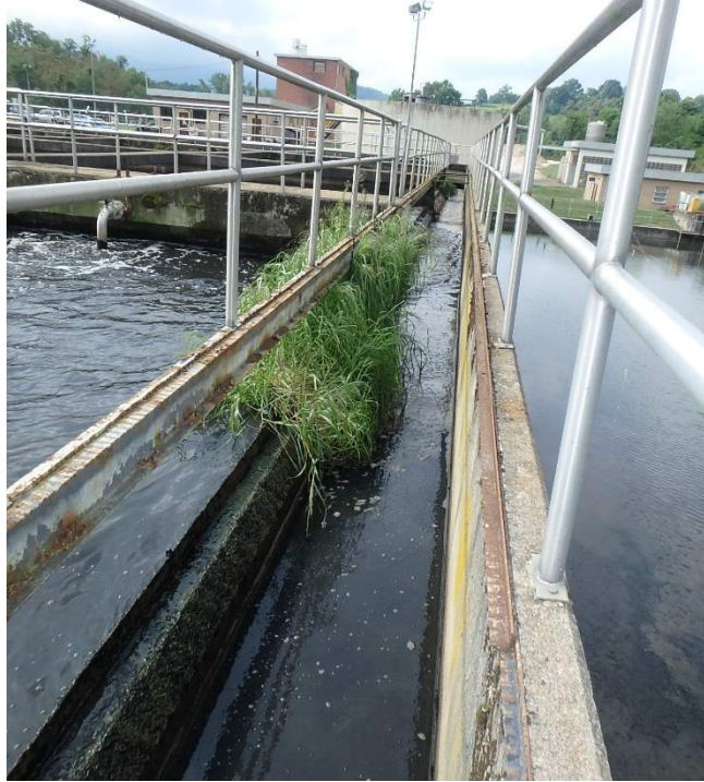
Figure 9. Drainage trough at west end of aeration basin. Original steel grate used for walking surface has been removed. Note substantial vegetative growth.
