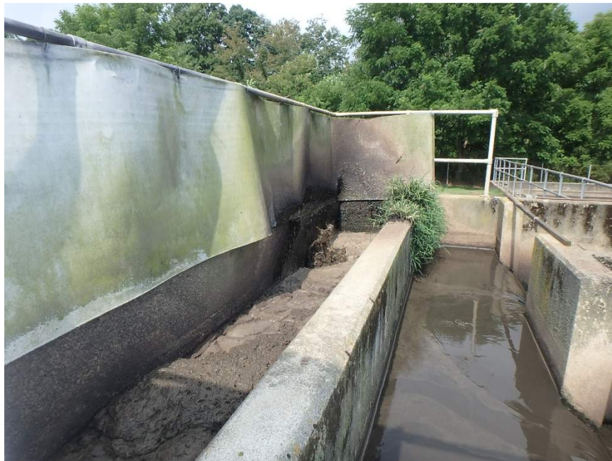
Figure 22. Sludge diversion channel at west end of secondary clarifier. Note vegetative growth.
