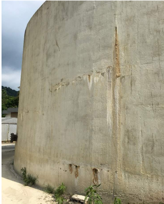
Figure 27. Cracks with efflorescence and corrosion staining at digester.
