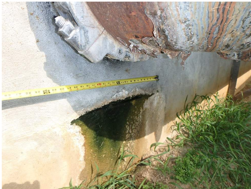
Figure 14. Crack with substantial leakage at east perimeter wall of aeration basin.
