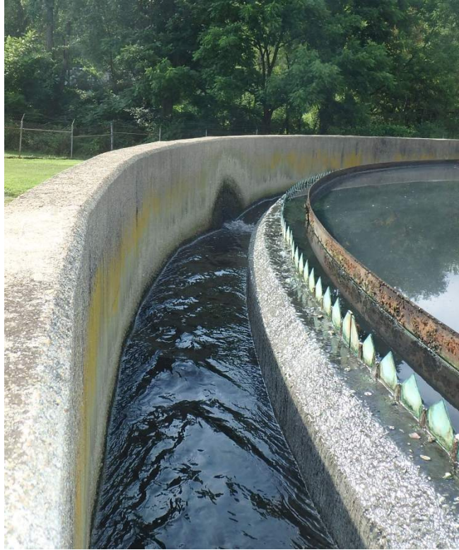
Figure 3. Annular drainage trough at primary clarifier.
