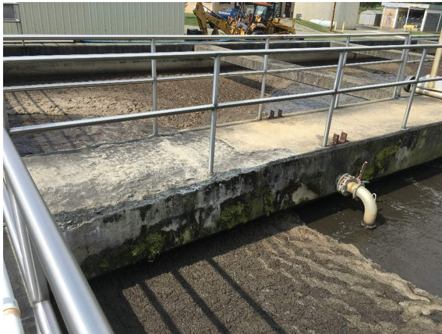
Figure 18. Widespread spalling and raveling of concrete at aeration basin walkway.
