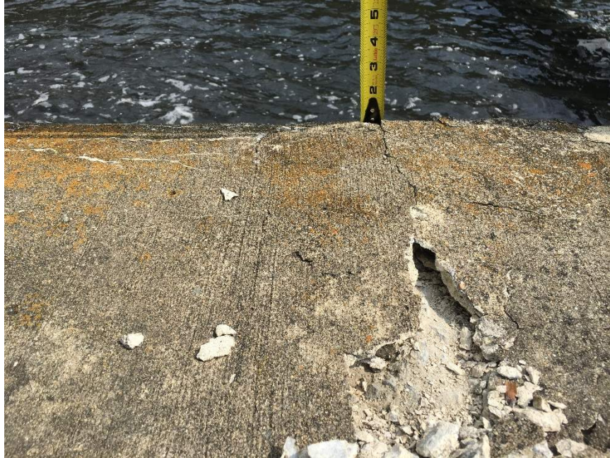
Figure 17. Localized delaminations and spalling at aeration basin walkway.
